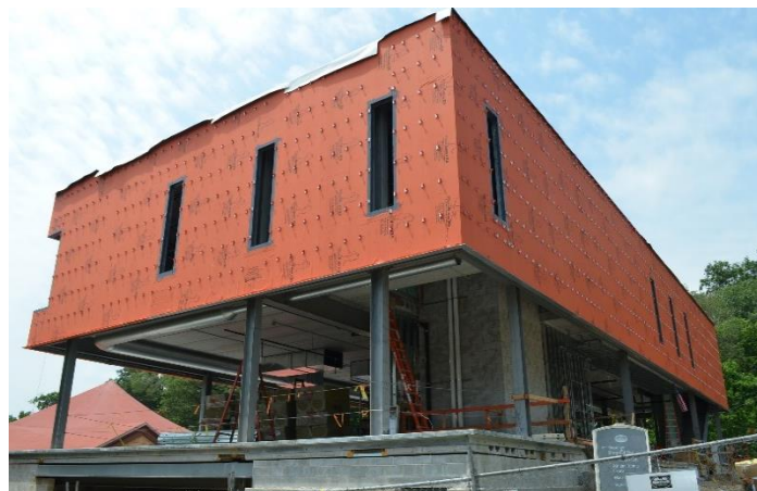
Over 9,000 sq.ft. of WrapShield SA Self-Adhered Water Resistive Vapor Permeable Air Barrier was installed on The Matchbox at Swarthmore College.
